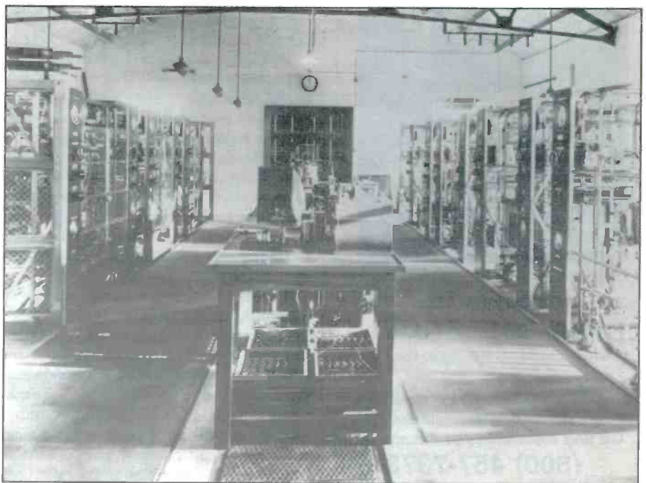
This is the transmitter room at the Marconi Beam Station, Tetney, shown in 1927. This station played a key role in popularizing shortwave as the primary medium for international communications. (Marconi Co. Ltd. photo)
