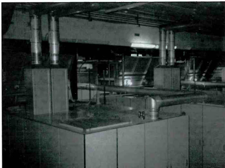
Here's a look at the 250-kW Collins transmitters at Sackville
