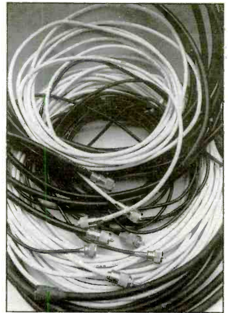
Spare coax cable sets are necessary to get signals out from underground shelters.
