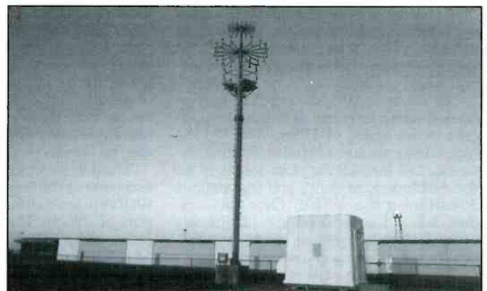
This view shows the full height of the radio direction finding antenna for the FAA at Grand Island, NE airport. (Sent in by Patrick Griffith, CO.)
