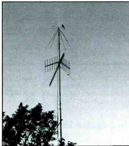
Discone antenna/bird perch above UHF corner-reflector yagi beam.
