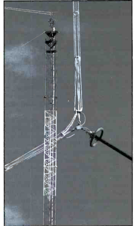
PART OF THE WWVB ANTENNA SYSTEM. Here's part of the WWVB antenna system—the connection point between the antenna downlead cage and the counterbalance insulator. The cage consists of six aluminum conductors mounted around rings approximately six inches in diameter. One of the support towers also is shown. While the WWVB and WWVL antenna systems are separate, they're identical. (Photo courtesy NIST.)
