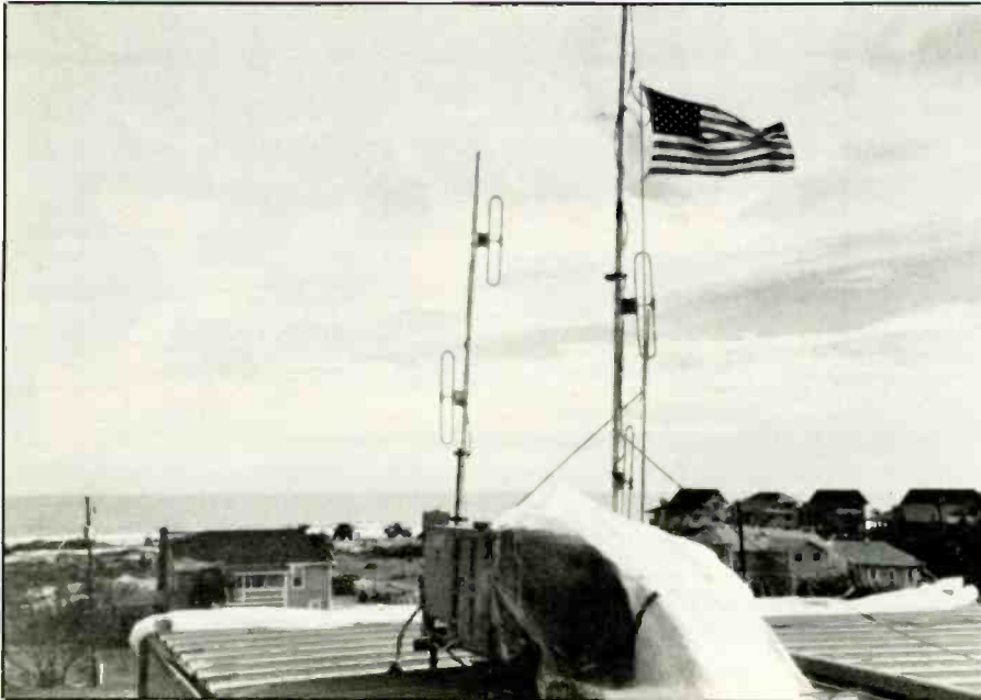
Disaster communications can be heard on scanners. This single base station antenna was left standing in a South Carolina town after Hurricane Hugo ripped through with 150 mph winds.
