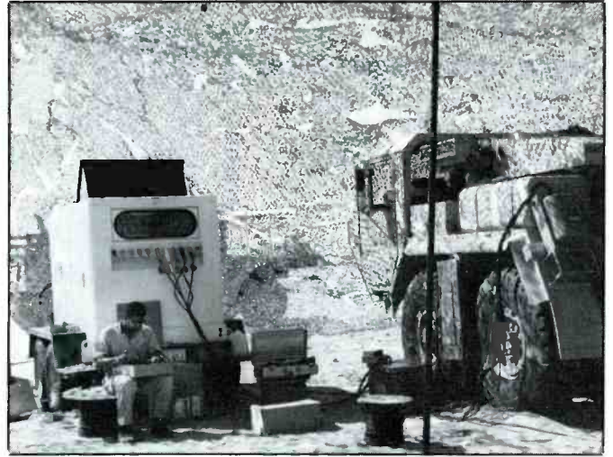
SFC Hosea Carlton USA, assembling power distribution panel at the 1st Marine Division site. Photo courtesy Capt. Jim Curtis USAF.
