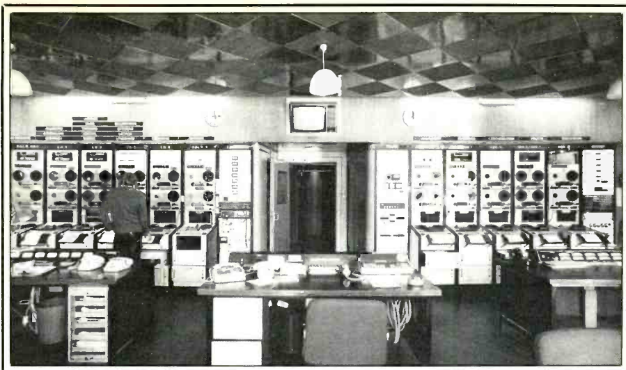
Master Control for both RFE/RL, from where programming is fed to transmitters in Spain and Portugal.
