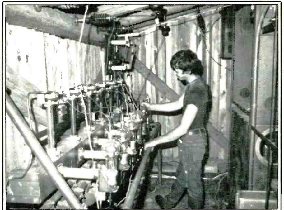
The main power supply for one of KPRC's AM transmitters is supposedly capable of putting out 10,000 volts!
