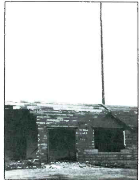
The El Salvadorian rebels secret communications center in this view reveals that the government located the station and took a decidedly dim attitude toward its operation. Oddly enough, they left the antenna and its' mast still intact!
