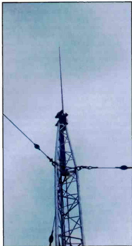
Parker's 20-foot tower, next to his new shack, supports a Clifton Labs Z1501D antenna.
