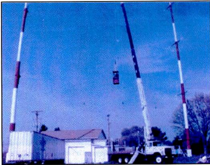
The WMLK tower in Pennsylvania being erected a few years back. (Courtesy of Charles Maxant)
