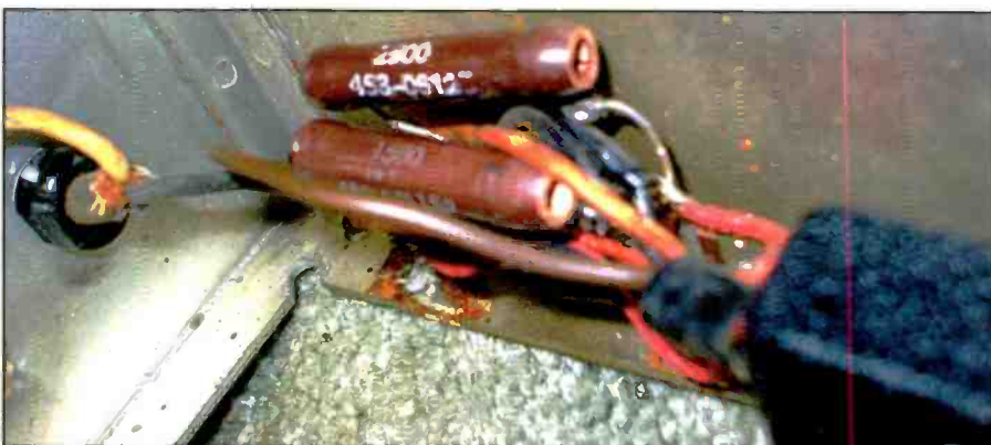
Photo M: The two tubular power resistors shown in this photo are not original and were installed too close to nearby insulated wiring.
