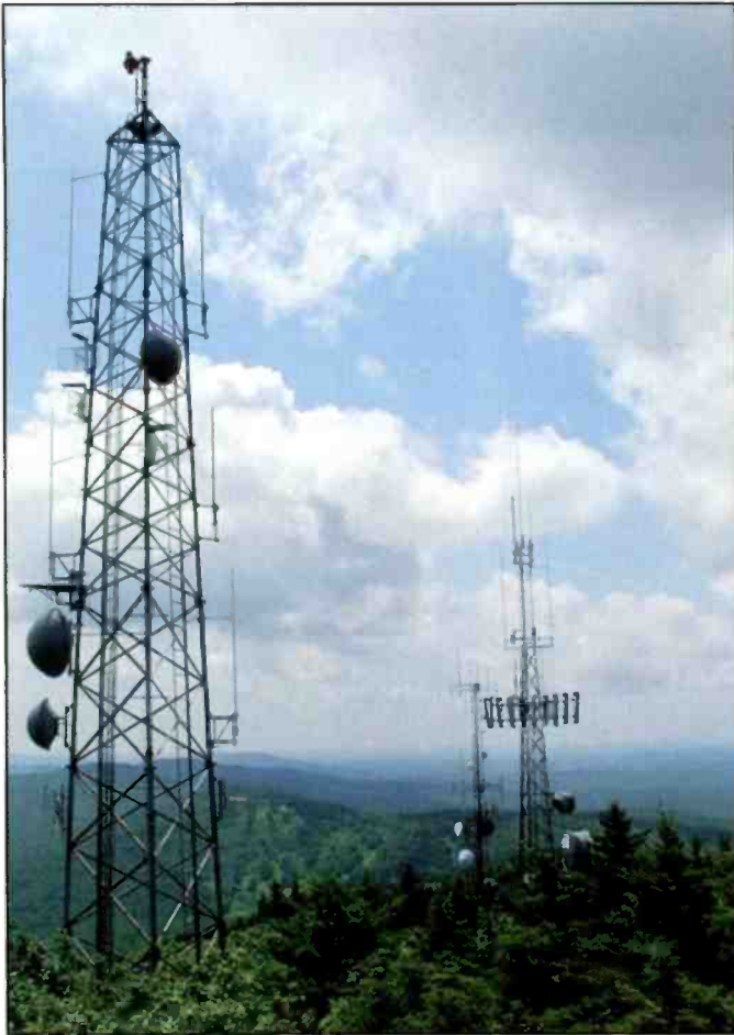
A radio station sale may require lease of the transmitter site, or sometimes only the "stick," or antenna. (Courtesy of Bruce A. Conti)
