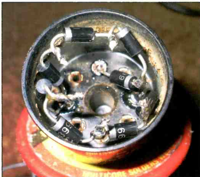
Photo D: Each side of the full-wave rectifier is comprised of four 1N5399 diodes in series for a total PIV rating of 4,000 volts. Note that modern avalanche mode diodes do not require equalization resistors or capacitors in parallel with each device.
