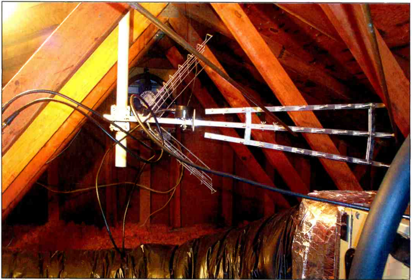
PHOTO 2: A high-gain antenna is positioned in the attic.
