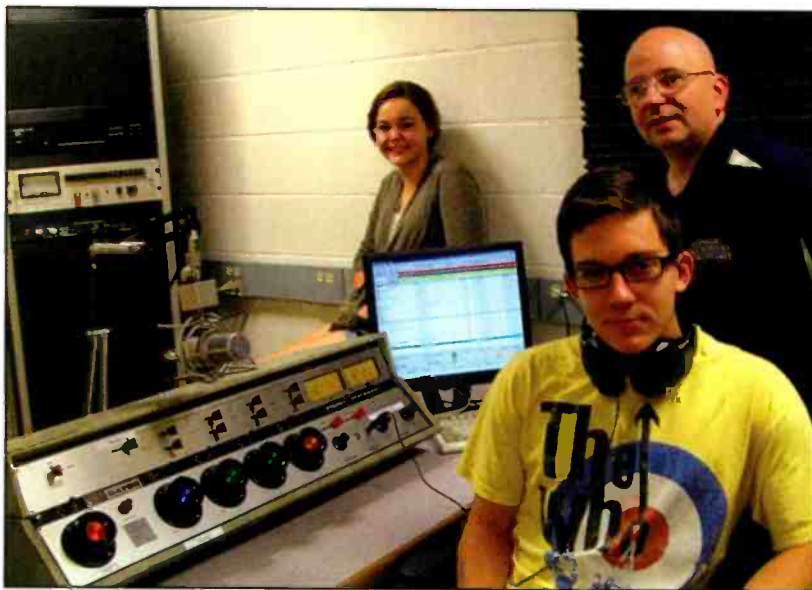
Here is the master control room for the campus radio station "McMahon FM" at Brien McMahon High School in Norwalk, Connecticut. Pictured is District Technician and Station Engineer Bill DeFelice, right, with students Anna Rae Newland and John Charles Moritz. (Courtesy of Bruce A. Conti)
