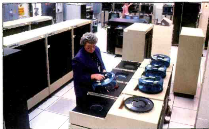
The environment is cool and clean in the PAVE PAWS computer room.
