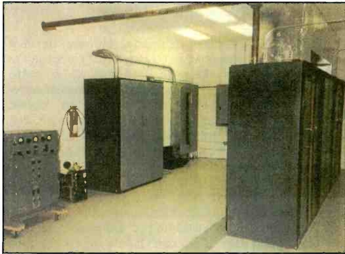
The transmitter and power supply at WRMI, Miami. (Thanks Charles Maxant, WV)
