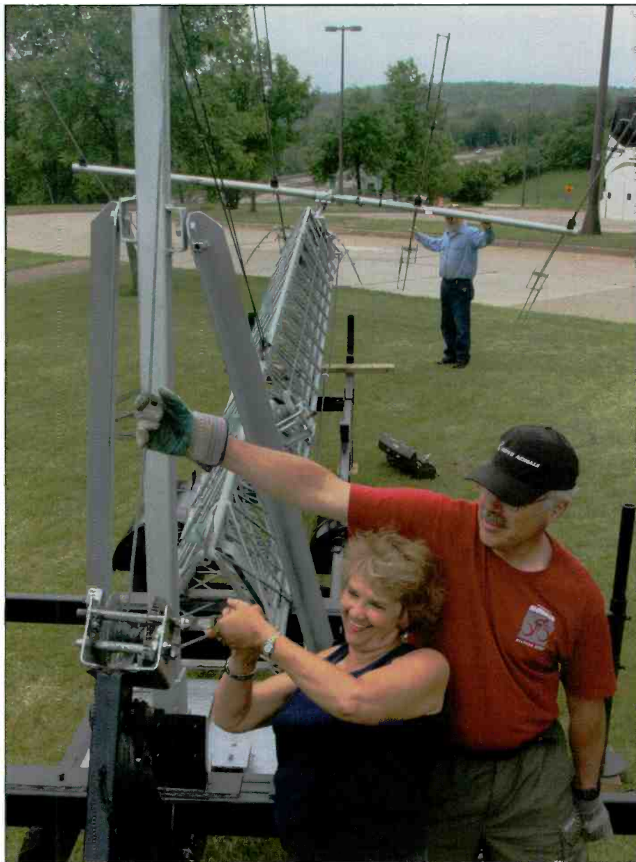
Teresa Dall, KAØCDO, and John Cavanaugh raise a 60-foot tower at a roadside rest area south of Duluth, Minnesota, for Field Day 2007. But what's wrong with this scene? You got it! No hard hats! (Photo by Paul M. Walsh via Wiki Commons)
