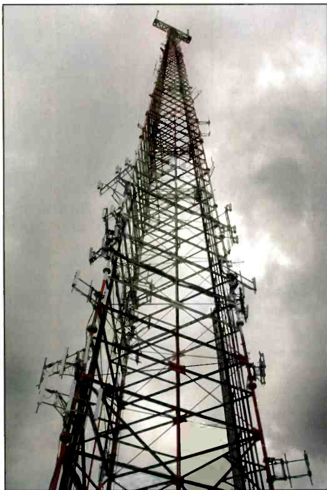
Antennas for the North Hills Amateur Radio Club's repeaters, including its D-STAR-equipped 70-cm rig on 444.350 MHz, are located on the tower of Pittsburgh's educational television station, WQED-TV (13). (NHARC photo by Bob Morris, K2RK)
