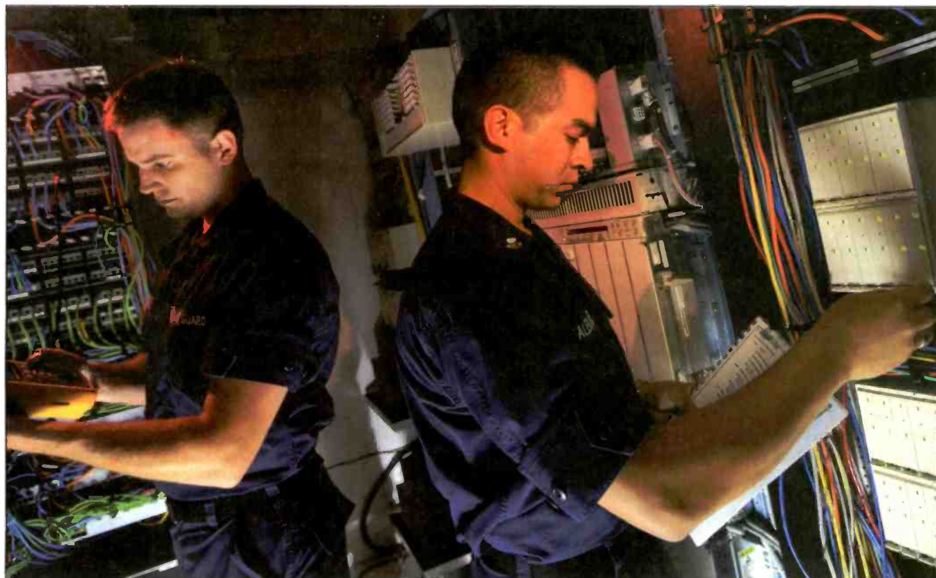
Two Coast Guard Information Technician Specialists working in a server room where information is stored and handled throughout the service.
