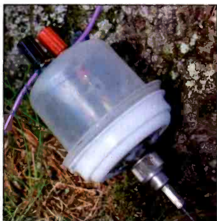
RF matching transformer assembled in a weatherproof food storage container.
