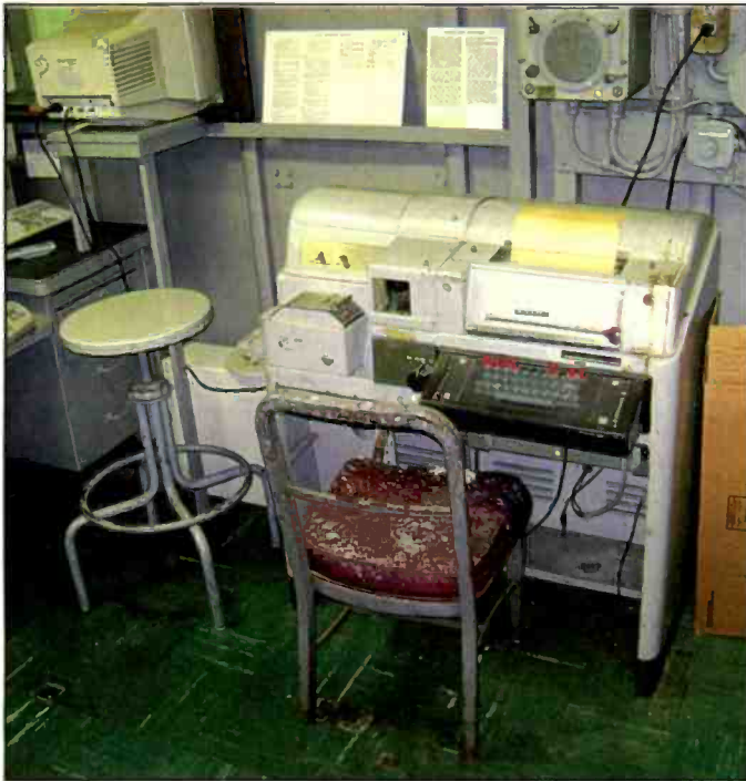
Photo D. Terminal for the AN/UCG-6 RTTY unit at W2PE aboard USS Little Rock used for RTTY contacts in the ham bands. (KC2HMZ photo)
