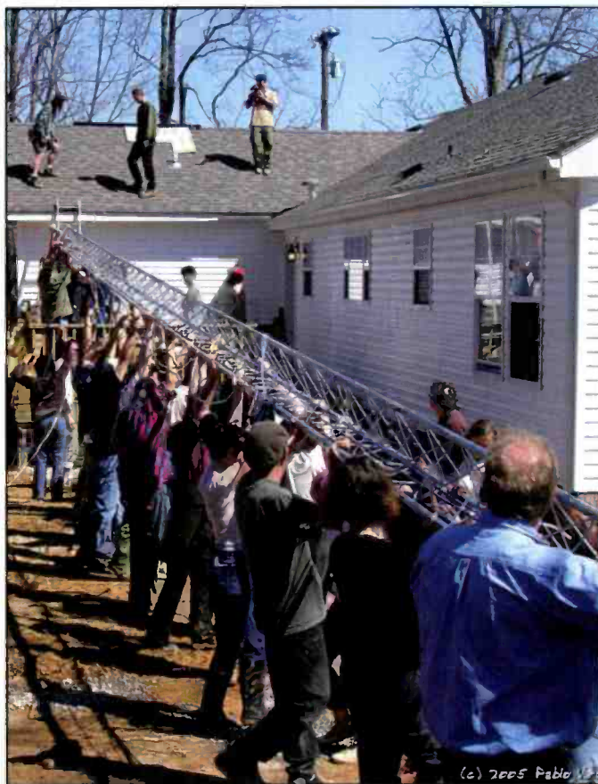
All hands were on deck to raise the tower on a Sunday morning at the WRFN-LP barn raising outside of Nashville, Tennessee, April 2004. (Photo copyright Pablo Virgo)
