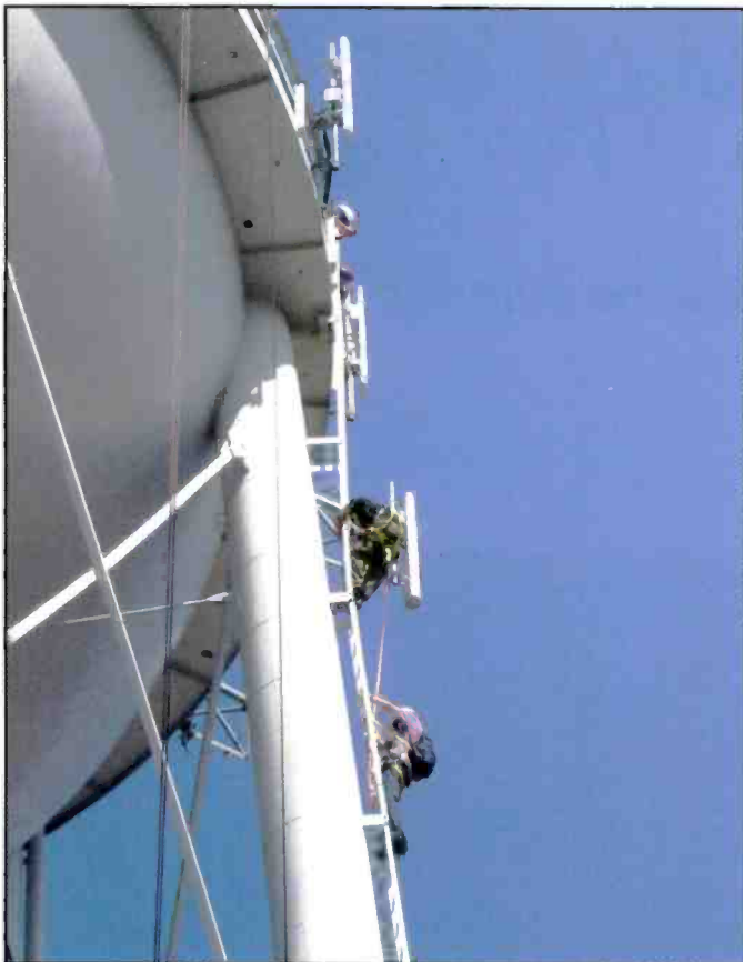
It was a long way up for the brave souls installing the antenna on the water tower in Woodburn, Oregon, at the KPCN-LP barn raising in August 2006.
