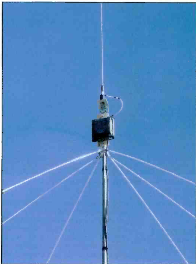
This long-range coast station SSB antenna system covers 4 MHz–26 MHz with the SGC autotuner. (Photo courtesy N9ZGE)
