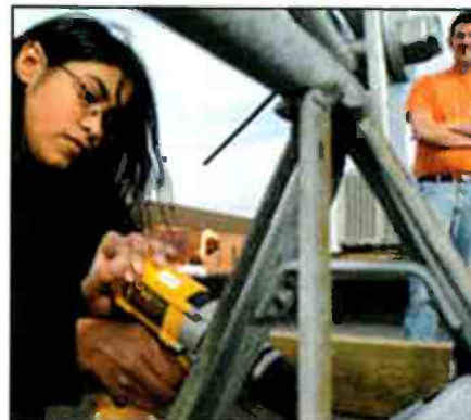
Securing mounting hardware for the tower at the WRFU-LP barn raising in Urbana, Illinois. (Photo copyright Jacques-Jean Tiziou)
