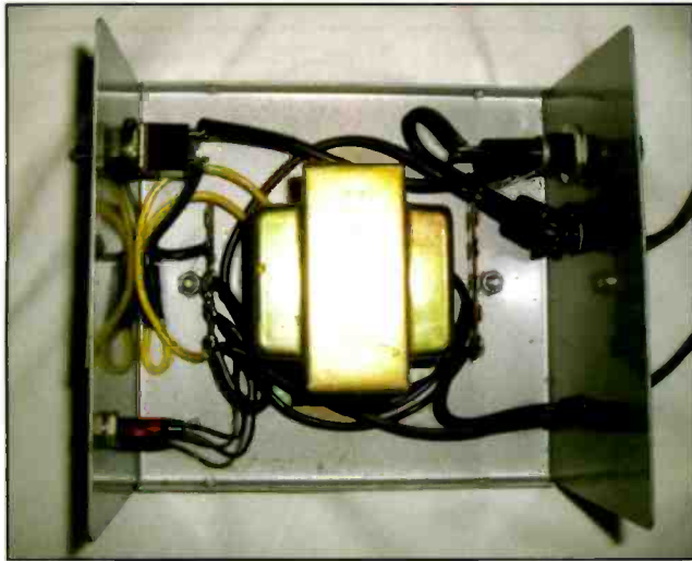
Photo C. Peeking inside shows that Ted's workmanship is clean and uncluttered. Good deal! Terminal strips are provided to support the internal leads and wiring, and the power cords are securely held as they pass through the walls using snap-mount grommets. These are the finishing touches that are the hallmark of a first-rate job.
