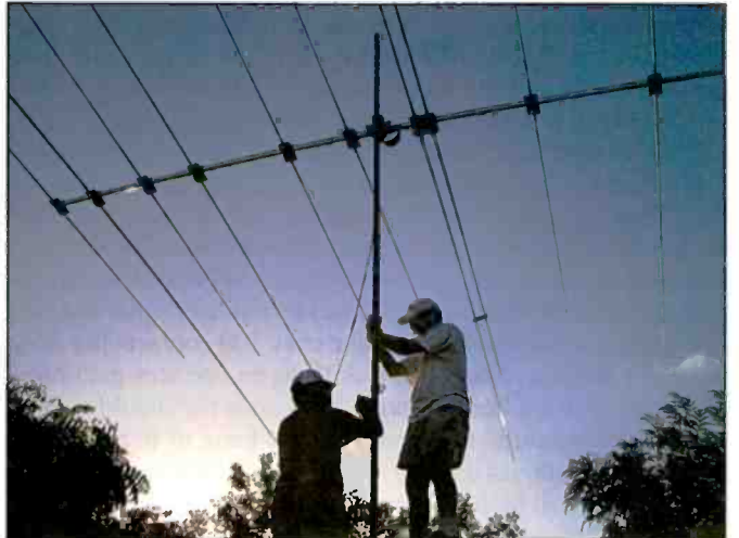
Bill Scholz, WIHIJ, and Dan Dankert, N6PEQ, put the finishing touches on a three-band HF Yagi at KP2AA (U.S. Virgin Islands). (Photo by Chip Margelli, K7JA)
