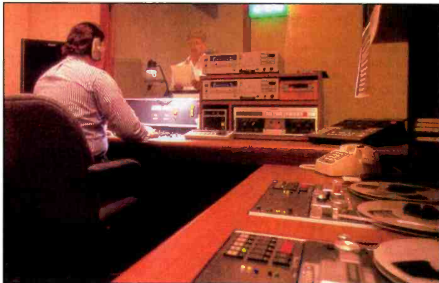
The control room at WEWN, Vandiver, Alabama. (Thanks Charles Maxant, WV)
