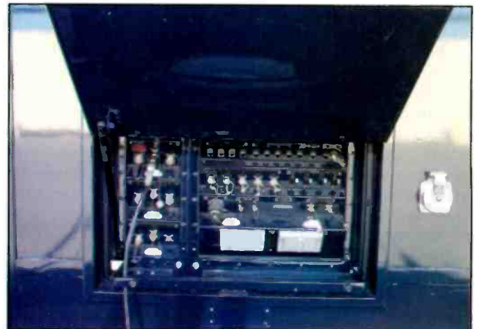
All antenna patching can be done outside the vehicle.
