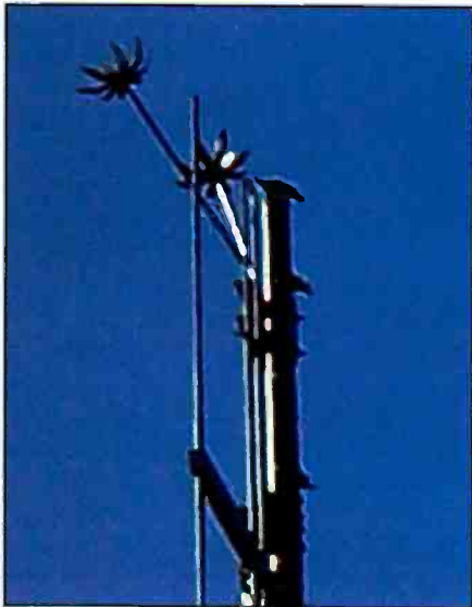
Photo H. Tower static dissipaters for lightning protection.
