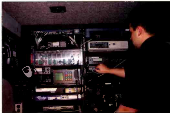
A peek inside the vehicle revealed plenty of radio equipment.
