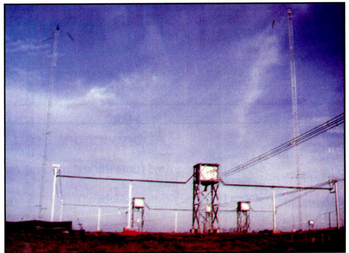
The antenna switching system at WEWN, Vandiver, Alabama. (Thanks Charles Maxant)
