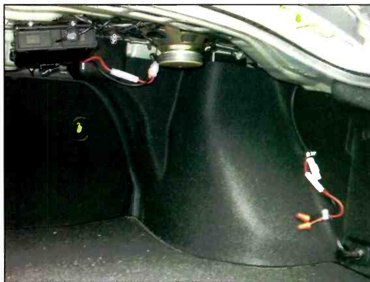
The DR-635T's main body is securely bolted to the upper portion of the trunk below the rear deck. Here, our cables haven't been completely protected with split tubing, but this view is shown to give you an idea of how out-of-the-way the main body is, even compared to the vehicle's factory-installed radio speaker, to the right. At the bottom right of the photo is the 12-VDC power cord plugged into the trunk's power receptacle.
