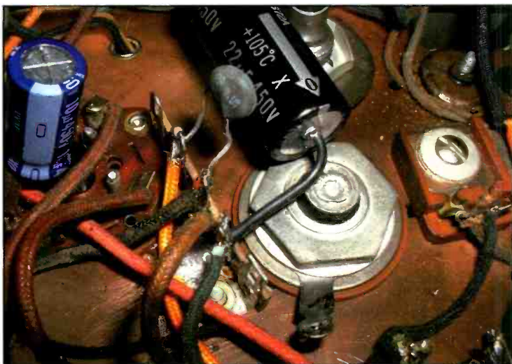
Photo D. Another ICL being used in a smaller Zenith tombstone chassis. These examples show how the devices are mounted away from nearby wiring or components. It should be well clear of the wooden cabinet baseboard when the chassis is back in the cabinet. Note the inch-long lead lengths on the ICL device and the firm mechanical connections.
