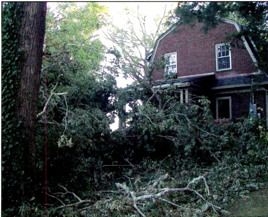
This photo shows a large oak tree that nearly destroyed a house. Had the tree fallen a few more feet towards the structure, that section would have been taken out. If you don't think it can happen in your neighborhood, think again—and be ready!
