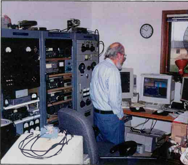
Here's a major Coast Station radio system in Alaska.
