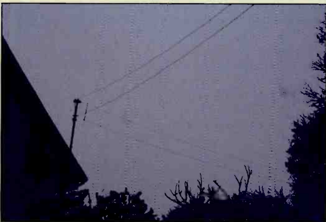
The shack end of the installation. The coax runs perpendicular to the antenna down the wooden pole and into the window to the right of the air conditioner.
