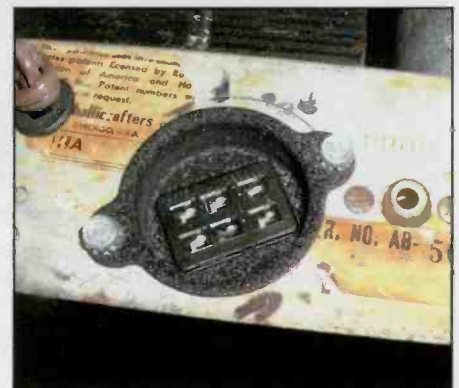
Photo G. The new accessory socket was mounted in the location where the power cord was previously located. The power cord was moved to a new hole and provided with a protective rubber grommet.
