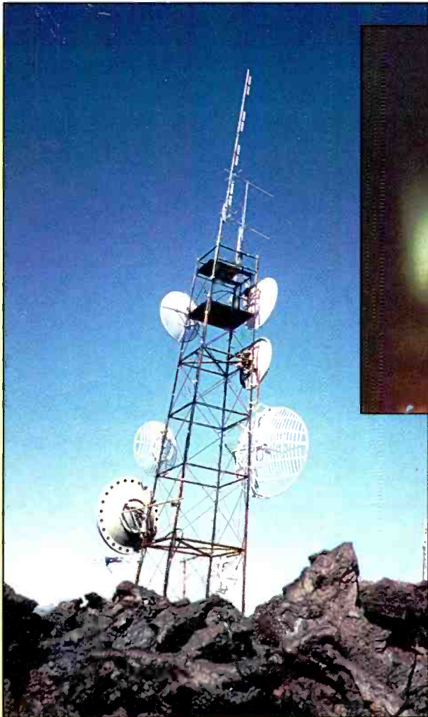
Hawaii's KH6HME 10,000 MHz beacon station. (Photo by Gordon West).
