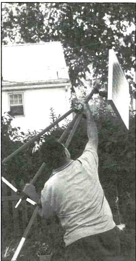
Standing the small Kyocera solar panel and single four-foot pole/ tripod assembly.
