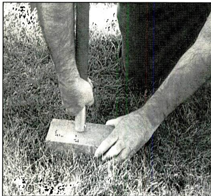
I decided to use a brick as a "base" for the center poles to keep the heavy poles from digging into the soft ground.
