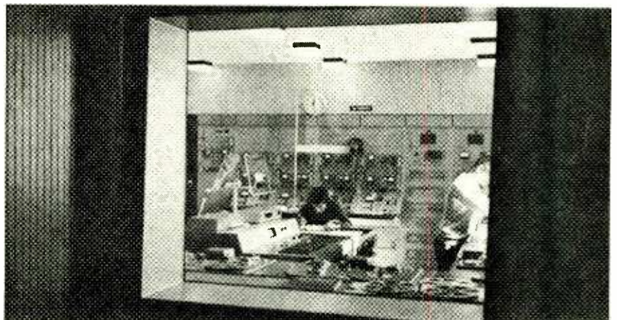
These two views show the inner workings of the shortwave relay station operated by Deutsche Welle, the West German international broadcaster, on the Mediterranean island of Malta.
