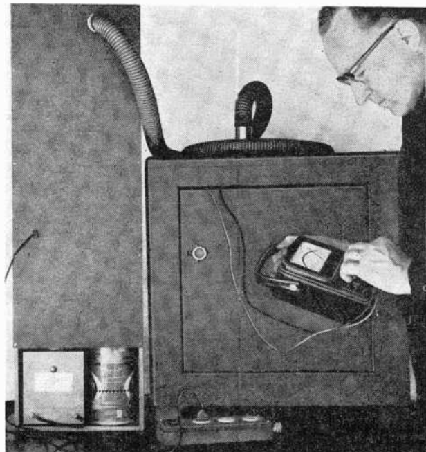
Fig. 9. The front door does not come down to the bottom of the cabinet to allow for air intake and observation of the indicator lamp. To prevent operation when the door is open, a TV "cheater" system is door operated.
