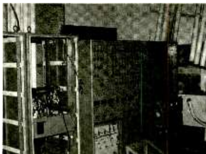
Now that's a circuit breaker assembly! This photo was taken inside the radar tower at Montauk. The two modules at the lower right appear to be power supplies. A bare rack seems to be loaded with cables that once connected to numerous modules. The abandoned site suffers greatly from disrepair and pillaging.
