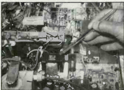
T105, the chopper-output transformer, is pointed out by the end of the pen. Q101 is mounted just to the left and on a vertical panel, with the Q101 terminals and socket side shown.
