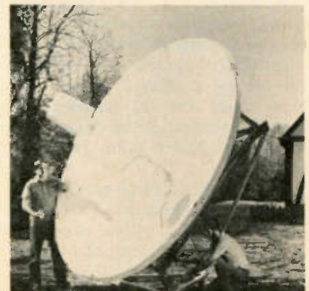
Figure 1 Installation of the antenna for the Heathkit Earth Station begins with the construction of three concrete piers for the steel foundation. The panels are then bolted together to form a parabolic dish that is mounted to the framework. The LNC electronic unit and its lines are mounted, and the entire assembly is tilted up and oriented to receive the desired satellite signals.
