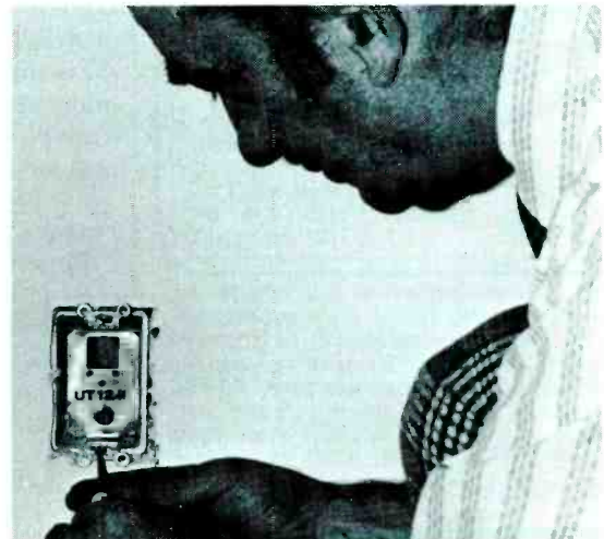
Fig. 3 Wiring is easier in some types of construction by the use of loop-through tapoffs. Each box serves both as a wiring point, and as a tapoff outlet for one TV.
