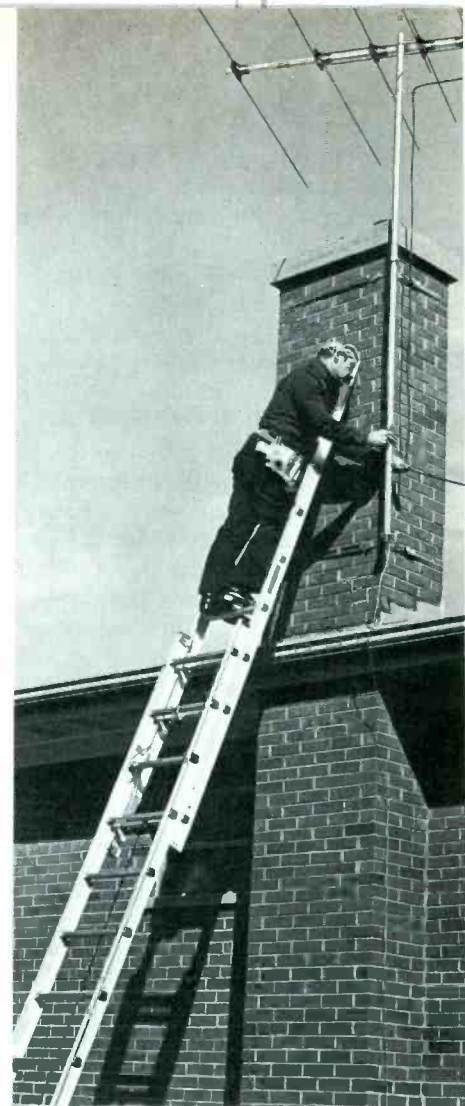
Fig. 1 Typically, an extension ladder is used for installations of outside antennas.
