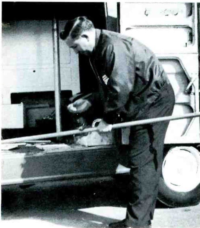
3:02 pm Cutting the 4' rotator mast from a 10' mast section using a plumber's pipe cutter. The plumber's pipe cutter produces a cleaner and quicker cut than a hacksaw.
