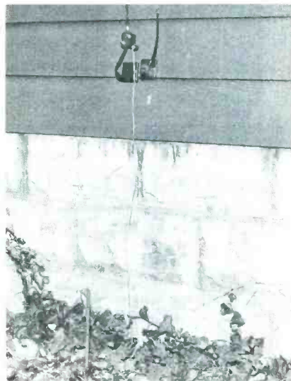
Fig. 5. The lead-in and rotator cable entering the house through suitable feed-through insulators. Before entering, the lead-in is fastened to a lightning arrester which is grounded to a rod.
