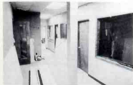
KJR's remodeling plans include new air, news, and production studios, shown under construction.
