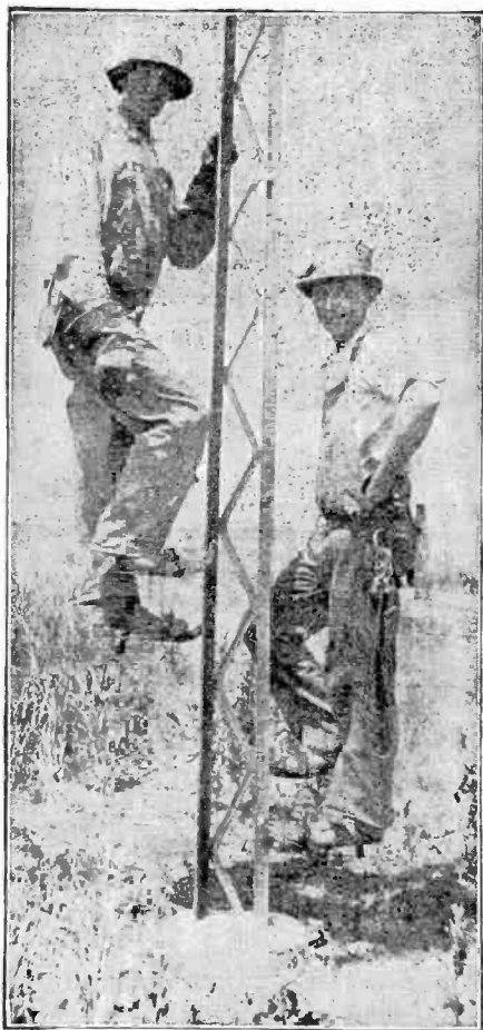
FIG. 5,804.—Erecting Bates steel pole 1. Pole as erected showing foundation, also a method of climbing by means of Bates pole climbers.
