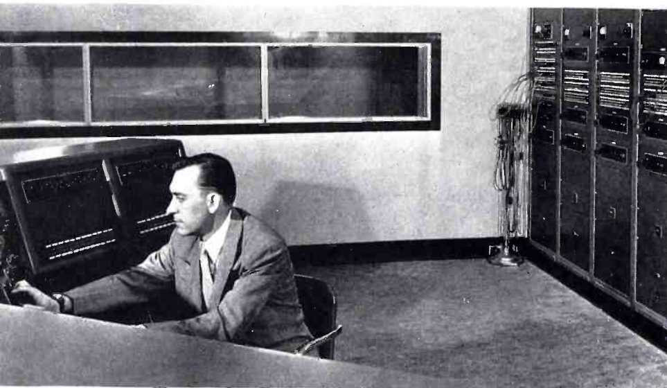
Racks in rear wall of combined master control-FM transmitter room put audio, test, monitoring equipment in easy reach of operator.
