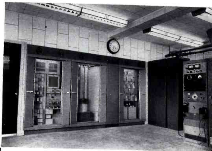
New operating room at KWK-FM for W.E. 10 kw FM transmitter.
