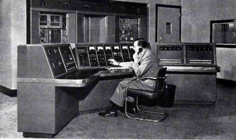
All program routing is done at RD100 console. Left wing holds order wire panel. FM transmitter is supervised from console position.
