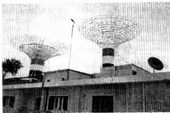
Fig. 3 The 100kW and 30kW Tanta CFAs situated on the same rooftop, separated by 6m (19.5ft)
