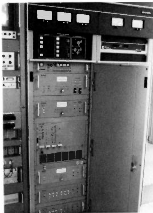
Figure 9 - Comark/Thomson-LGT Modulator linearity corrector in its exciter cabinet
