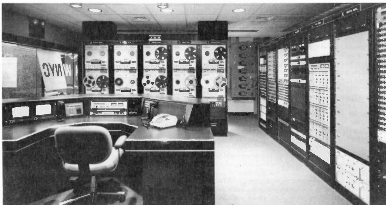
Figure 3. View of Terminal Room from monitoring console. The reception room vision panel and WNYC logo are at the left. Mounted on the wall between the tape machine and equipment racks are the HVAC controls.
