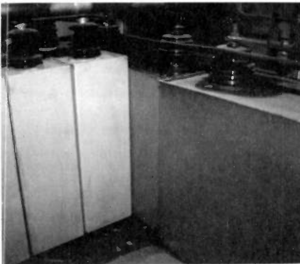
A Leaking Large PCB Capacitor
