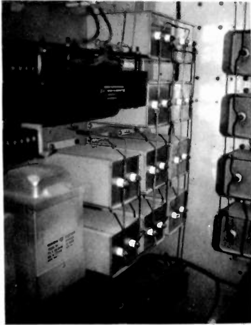
Small PCB Capacitors in Rectifier Cabinet
