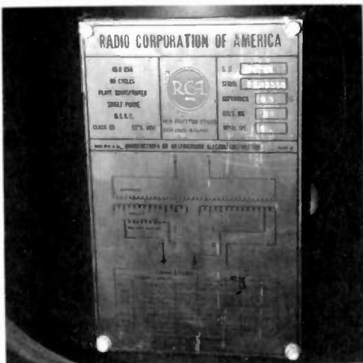
Mineral Oil Transformer Nameplate
