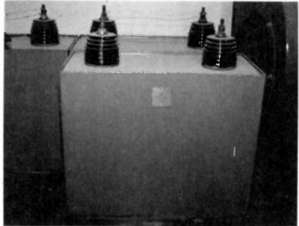
Spare Large PCB Capacitors
