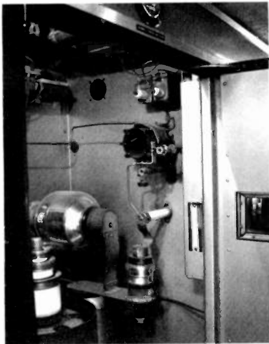
Small PCB Capacitors in Power Amplifier Cabinet (upper right)
