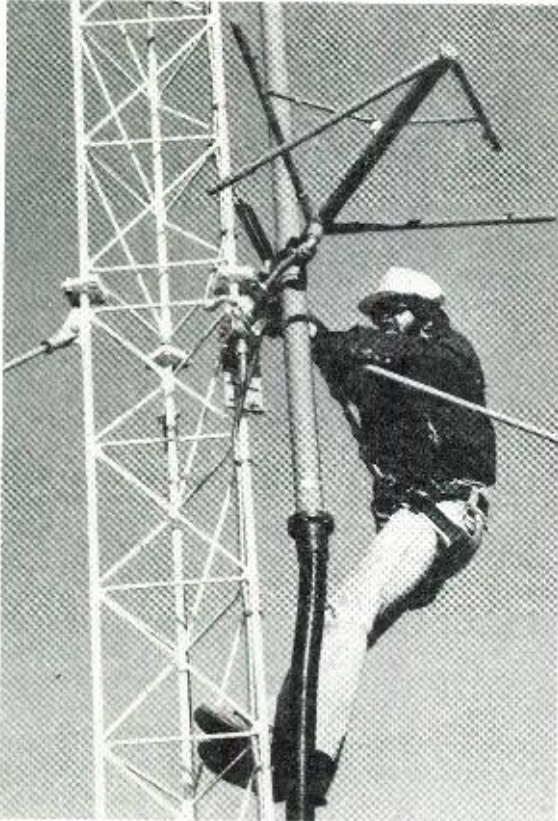
Fig. 21. Rigger finishing electrical tie in box for deicers. Looped stainless steel heaters were factory installed in the four arms, plus one in the feed support boom. (Photo courtesy Cetec Antennas)
