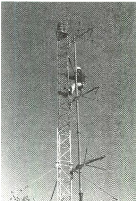
Fig. 9. Three bay Cetec model JSCP-3 non-symmetrical FM antenna mounted on the tower leg. The guy cables are insulated fiber glass rods near the tower legs. (Photo courtesy Cetec Antennas)
