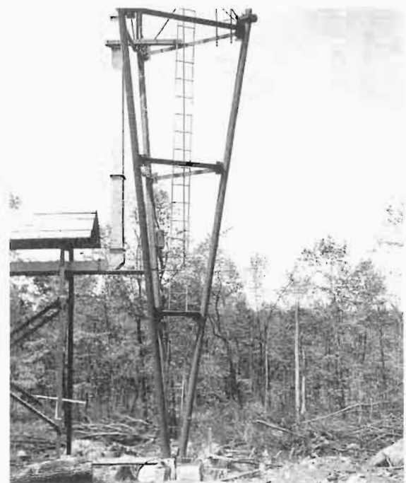
Fig. 6. Photograph showing tapered-base type tower.
