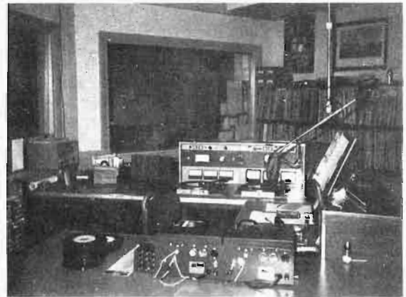
Fig. 7. Broadcast control room and announcing studio.
