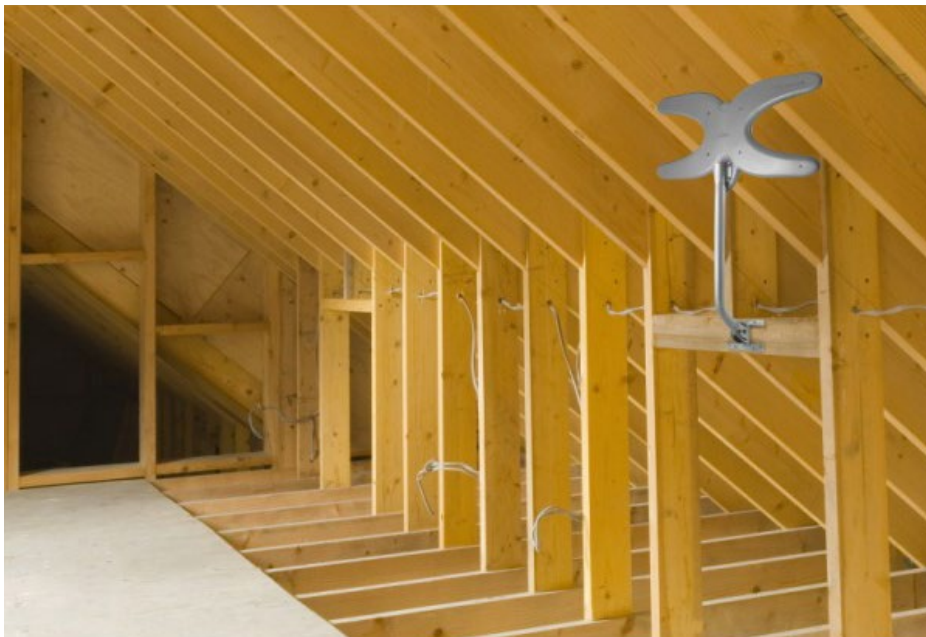
Attic-mounted SKY antenna (Courtesy: Mohu)
