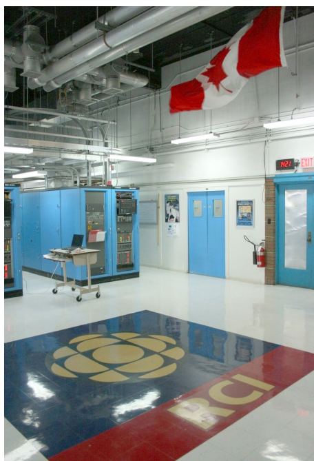
Interior RCI Sackville Transmission site.
