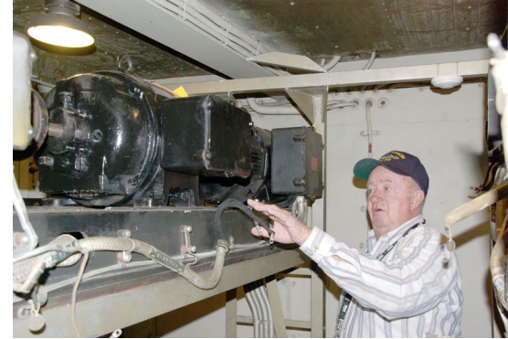
Norm showing the generators.
