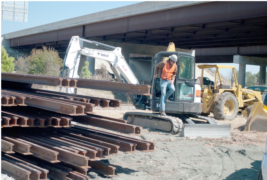
At the so-called Hopson Road project between Durham and Raleigh, North Carolina, contractors are just starting to stage their equipment and supplies in early April of 2013. This project involves a curve realignment (for faster passenger train speeds) and the addition of a passing siding for the railroad and a grade-separation for crossing with busy Hopson Road. Rails have already been brought in, but these are relatively light rails. With new construction, such as new sidings, the new tracks are sometimes built with lighter rails, which are then swapped out for heavier rails once on-track equipment can be brought in.
