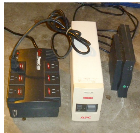
Photo B Daisy Chained UPS
