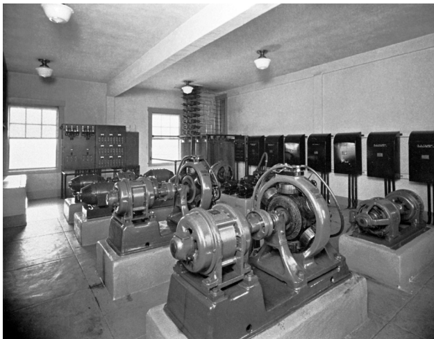
The generator room of the General Electric station contained nine motor-generator sets. These supplied current for heating the filaments of the tubes, plate potential for the power amplifiers and the 600 meter commercial transmitter, bias potential for the amplifier and modulator tubes, and excitation for the various generators. These machines were all in duplicate, thus assuring a continuous program in the event of failure.
