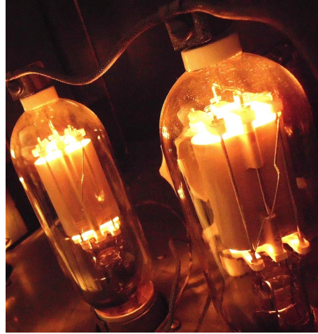
The tubes are kept glowing for visitors in the power supply for the museum’s 5 kW AM broadcast transmitter from the 1930s.
